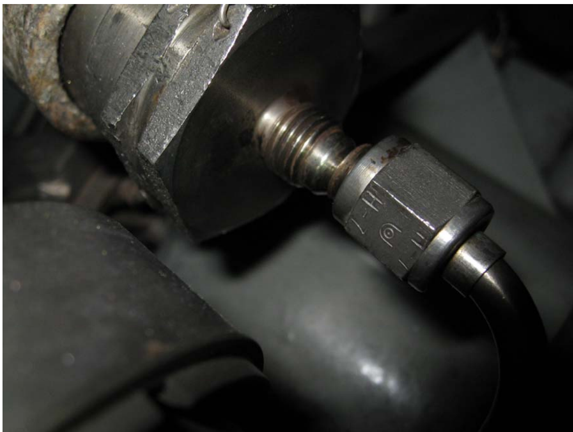
Figure 5. A B-nut downstream of the Pc filter on the compressor delivery air pressure sensing line, photographed after the accident.
