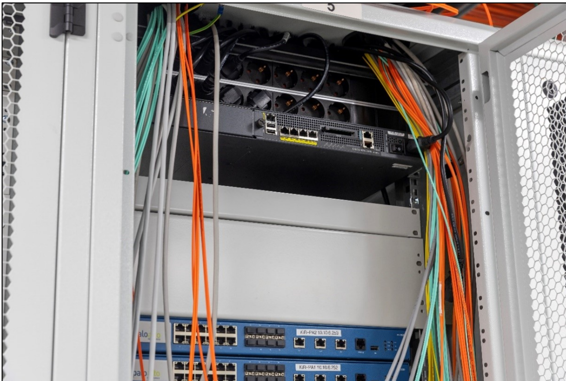
Figure 7. Hardware cabinet at KASKO's data centre in October 2024. The image shows the backup VPN device ASA 5545, which was never commissioned. ASA 5515, which was used in the data breach, was located below it.
