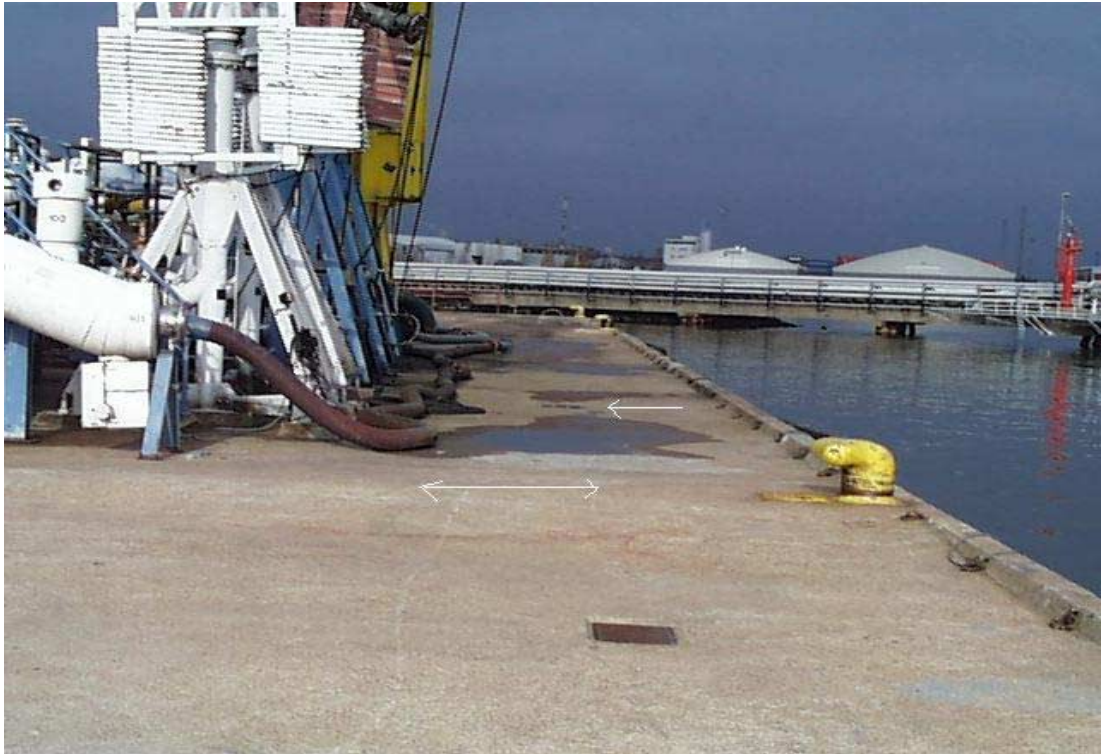
Figure 5 Upper one-way arrow points at the drain at the actual loading area leading to the pier well. The two-way arrow points at the platform that separates the loading area from the rest of the pier.
