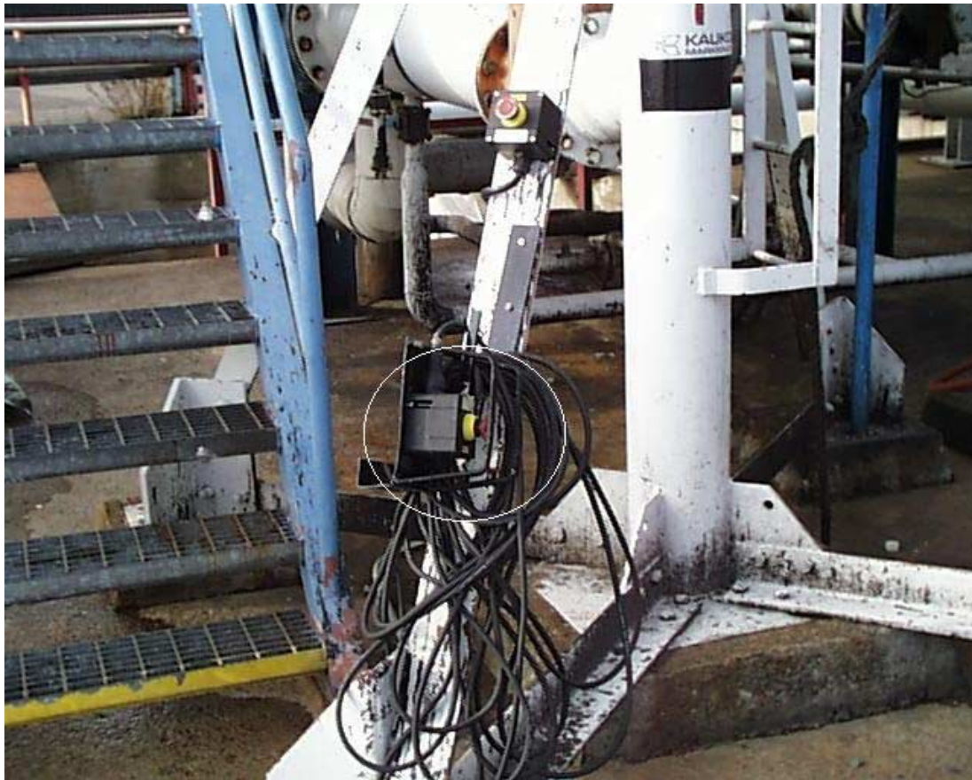
Figure 14 Cabled emergency stop button of Kaukomarkkinat for loading pump (circled). Can be attached on the railing of the vessel. Installed after the overload of the CRYSTAL RUBINO.
