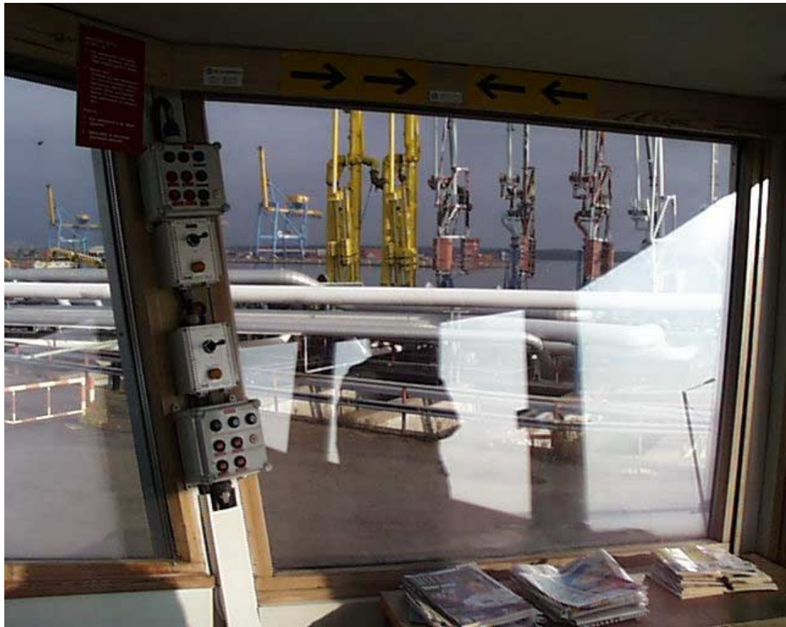
Figure 13 Limited view from the pier control room to the ship. Left in the picture the remote start for fire pumps and controls for fire cannons
