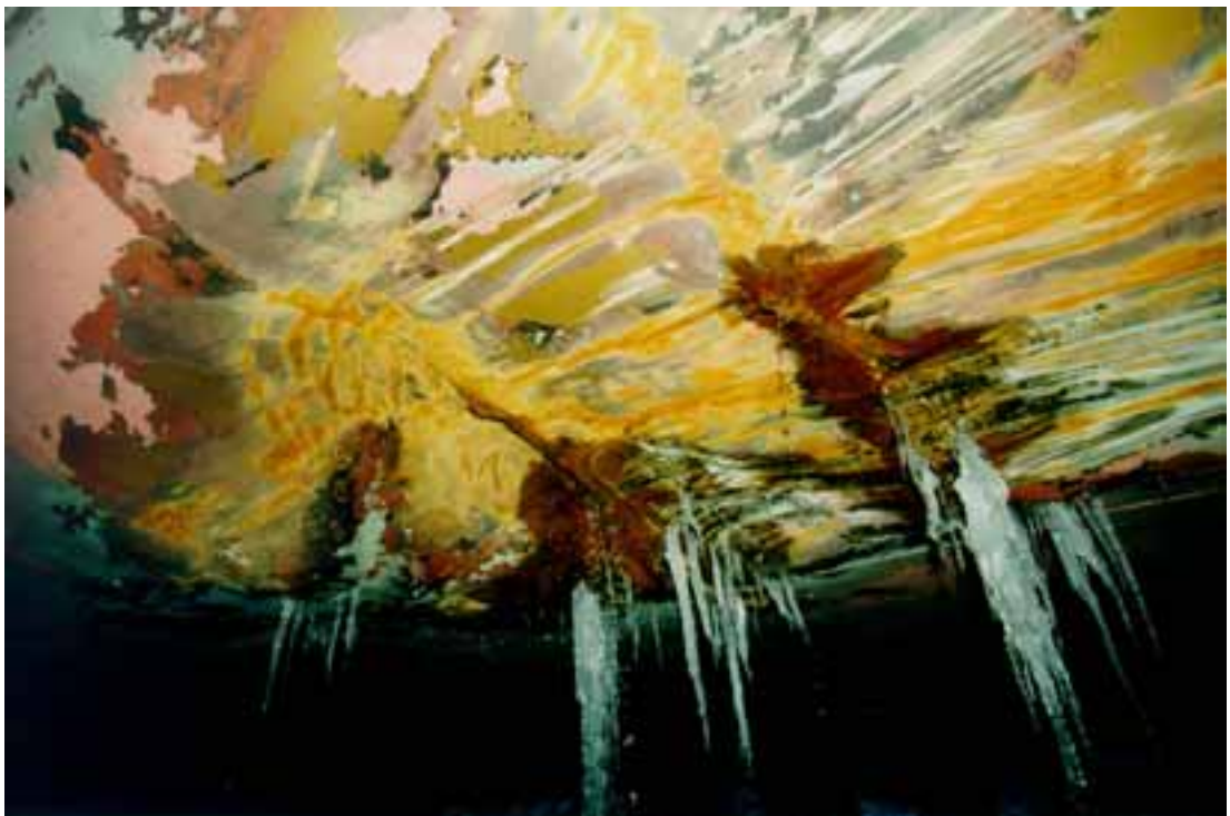
Figure 11. Hull damage on outer bottom of vessel. Water dripping out of a ballast tank
