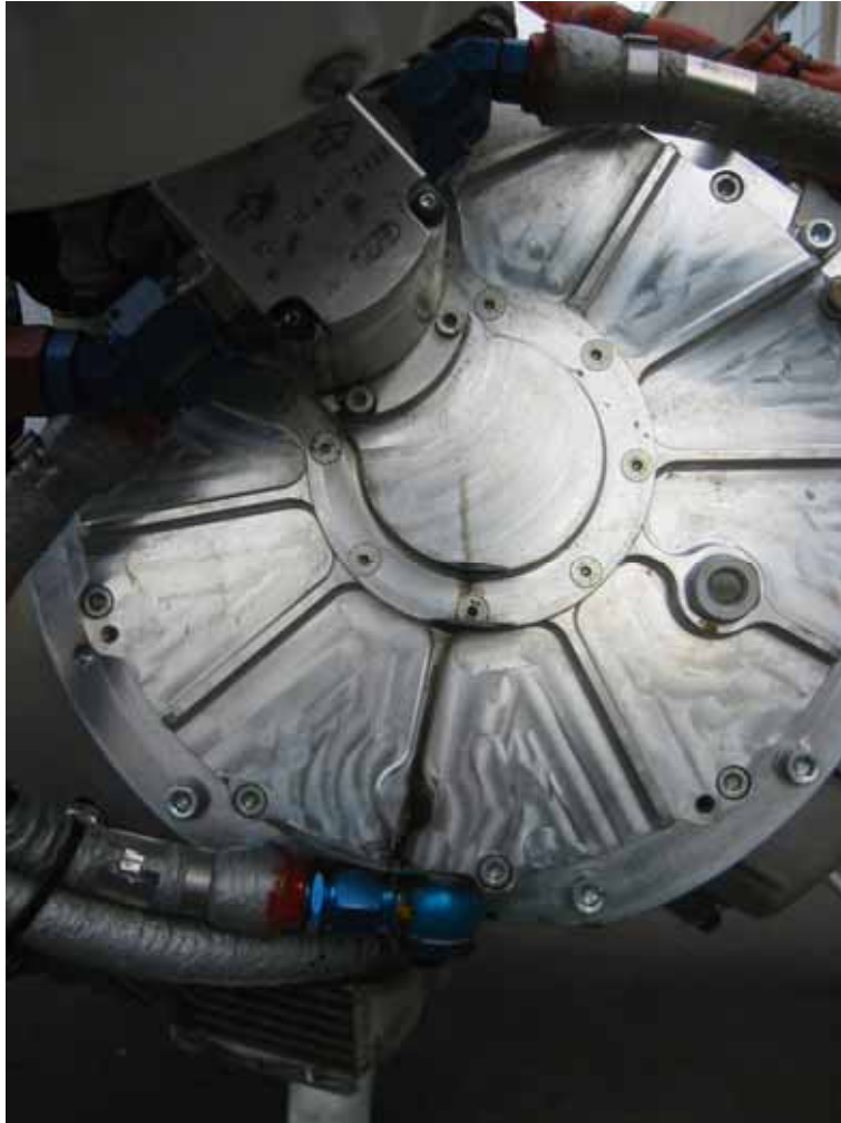
Figure 7. The oil leak from the Combi pump ran down the front of the gearbox onto its lower edge, from where it dripped into the inside front of the lower engine cowling.
